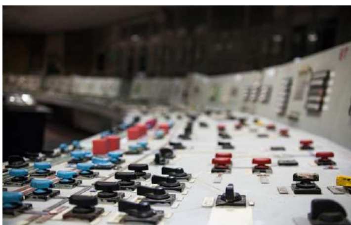
Figure 10-3. Nuclear power plant control panel
